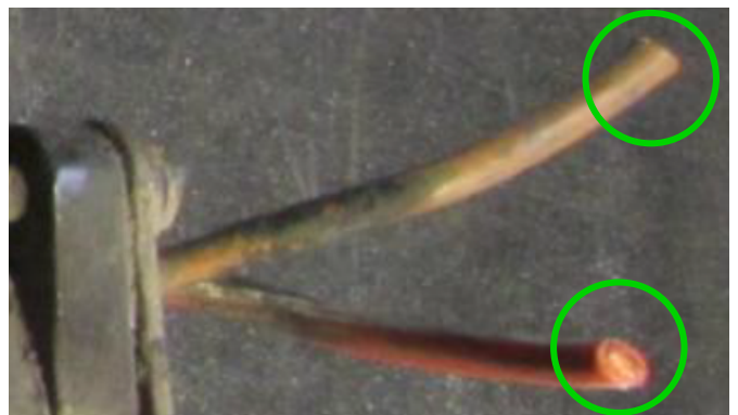
Cut or damaged cables
