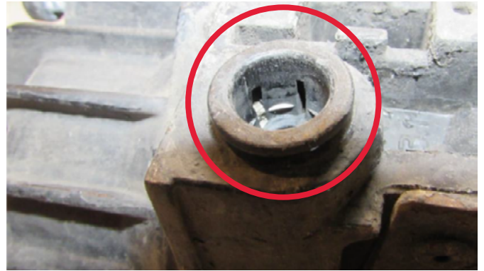
Missing components. Corrosion inside.
